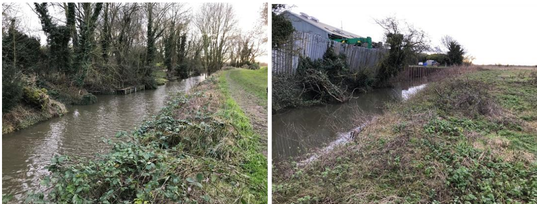
Plate 11 Uniform character of Catch Water Drain (left), and sheet piling along left bank (right)
